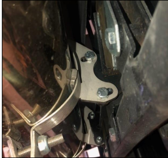
Figure 50: Muffler brackets loosely installed.
